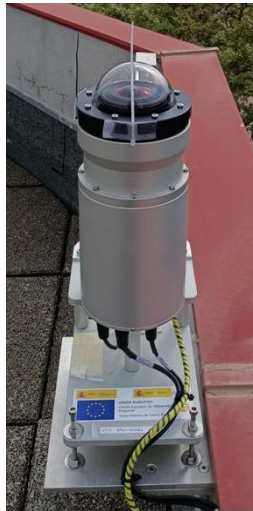
Figure 50. Outdoor installation: materialisation of the West direction on the camera body.
