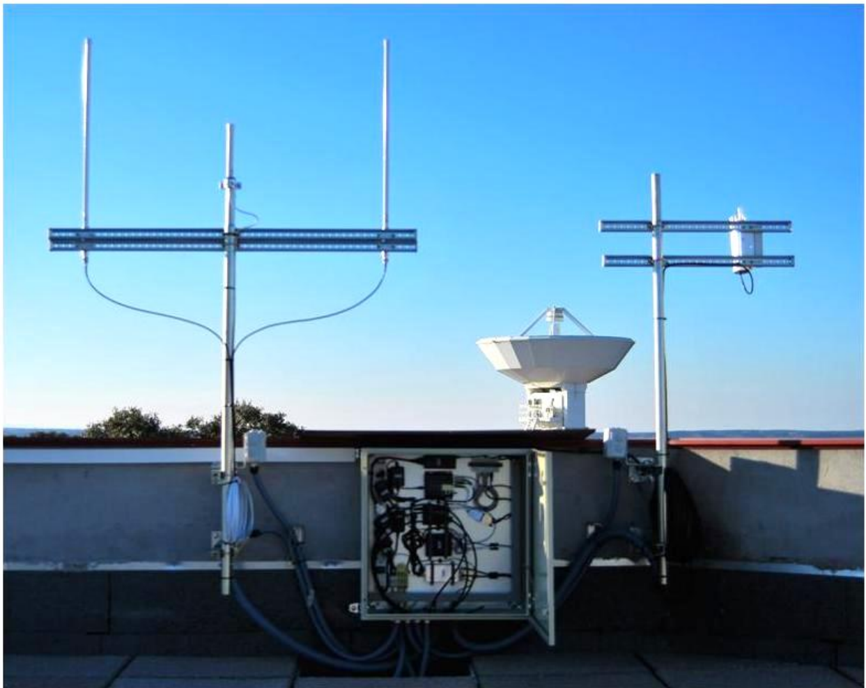
Figure 34. Outdoor installation: general view.
