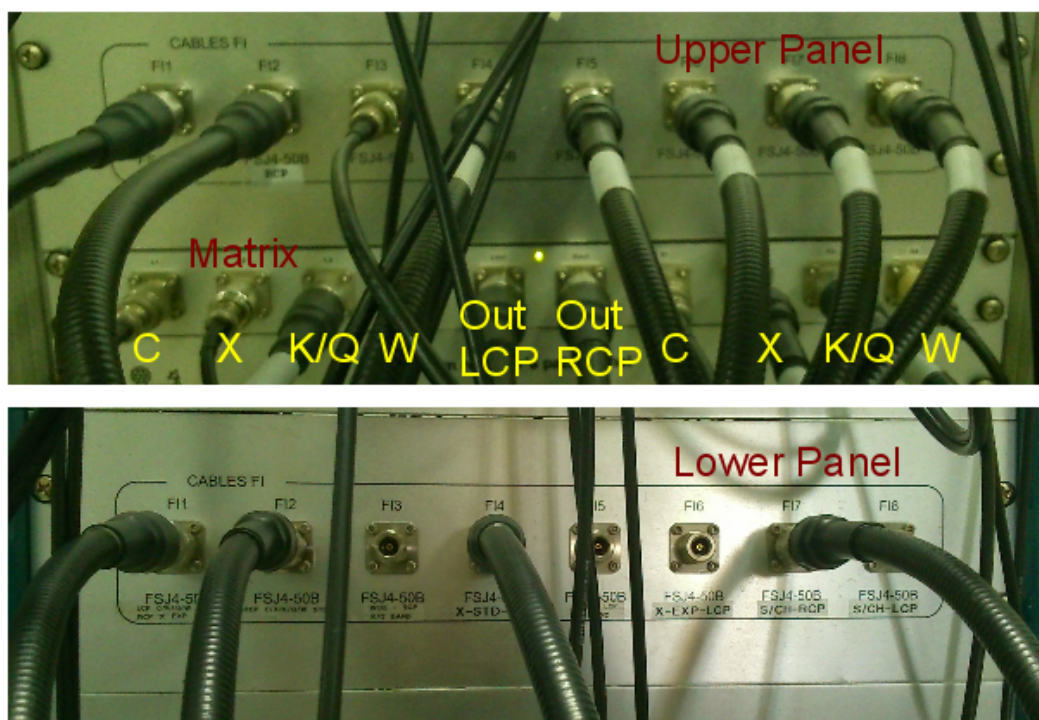
Figure 1: From top to bottom: upper patch panel, switch matrix and lower patch panel.
