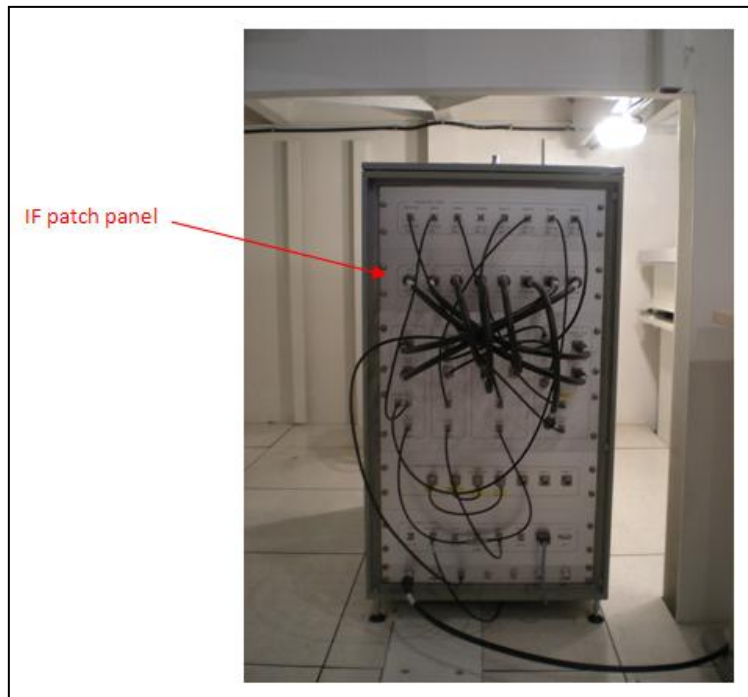
Figure 1: Receiver's room patch panel
