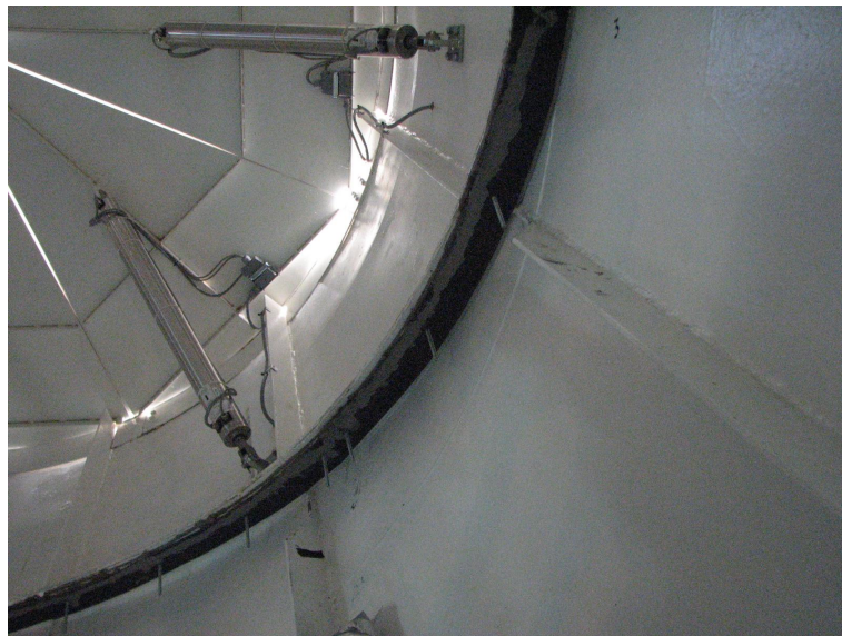
Figure 5: The mounting bolts on the steel ring.
