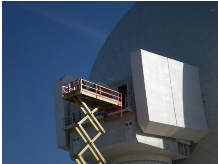
Figure 6: The new membrane was lifted on the telescopic platform and taken inside the receiver cabin.
