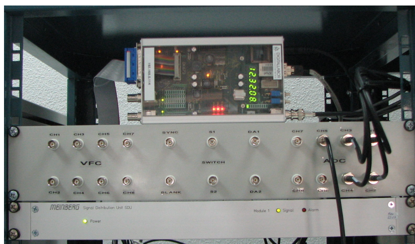
Figure 3: Current installation of the PBE in a rack in the Backends room. The PBE stands on one of its sides, so that the LEDs on top of the device area easily visible.
